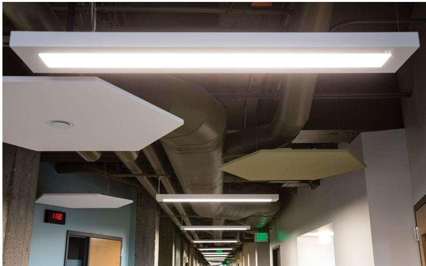
Enlighted Luminaire Level Lighting Controls installed in the Pacific Tower building in Seattle, Wash.
