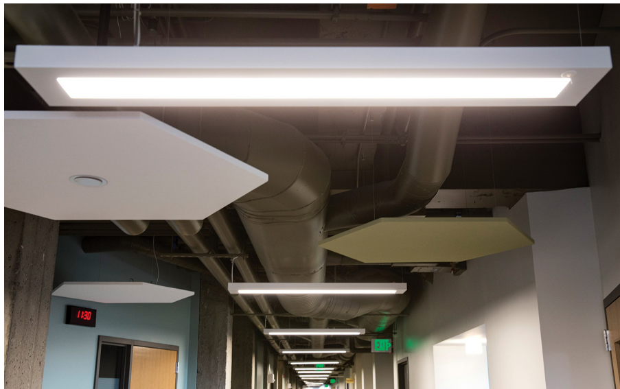
Enlighted Luminaire Level Lighting Controls installed in the Pacific Tower building in Seattle, Wash.
